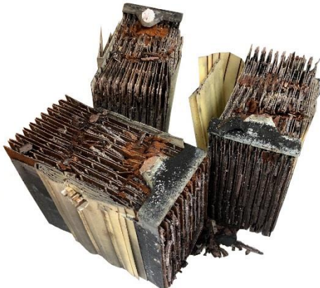
Three 2-volt cells from the original battery
